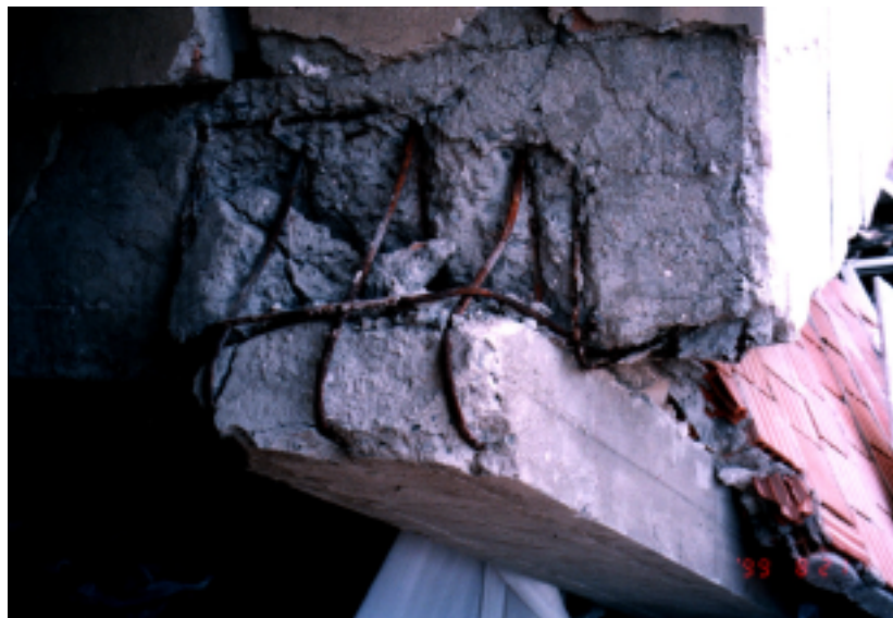
Figure 9.3 Improper column-beam connections (Note that reinforcing bars have smaller diameter and are not hooked with each other and lack of stir-ups and also lack of adherence of concrete. The building is shown in Figure 9.14
