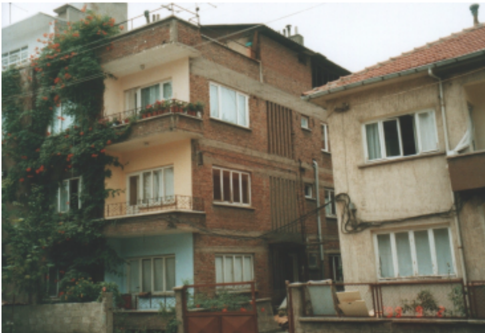
Figure 9.8 Non-damaged buildings made with solid bricks in Tıncalılar district of Adapazarı where liquefaction was widespread
