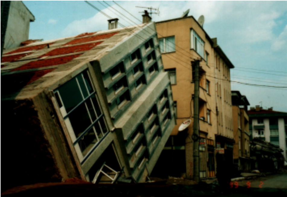
Figure 9.7 Toppled and collapsed buildings in T c lar district of Adapazar
